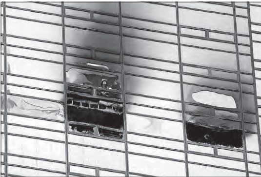
A firefighter looks out from the window of a fire-damaged apartment in Trump Tower, on Saturday in New York. The Fire Department says the blaze broke out on the 50th floor shortly before 6 p.m. Saturday. [CRAIG RUTTLE/THE ASSOCIATED PRESS]
