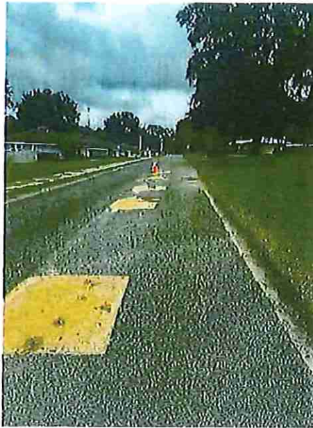
Photograph 1. Overview of Previously filled areas with additional subsidence.
